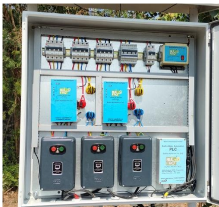
Bulfro PLC & water automation control panel
